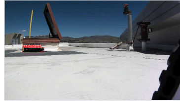
f Debris And Vegetation (Medium)
