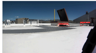
c Debris And Vegetation (Low)
