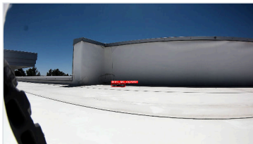
e Debris And Vegetation (Low)
