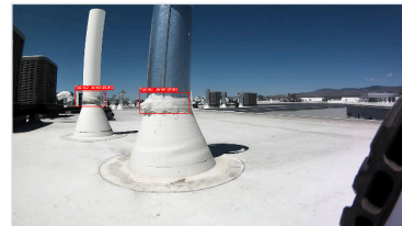
c Flashed Penetrations (Low)
