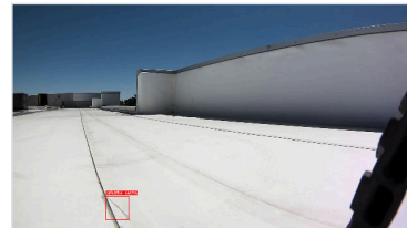
c Defective Seams (Low)
