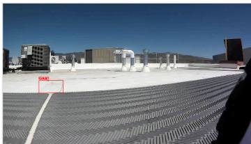
d Patching (Low)
