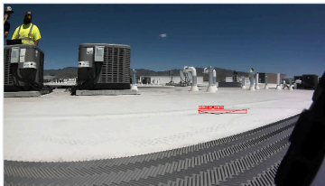
a Defective Seams (High)
