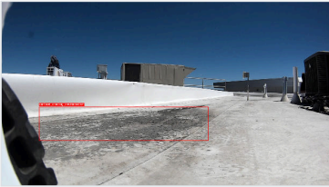
a Surface Coating Deterioration (Low)
