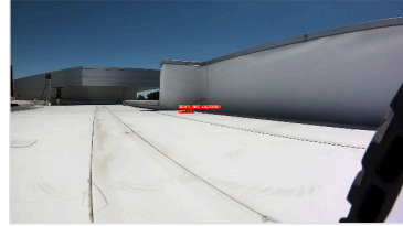
c Debris And Vegetation (High)
