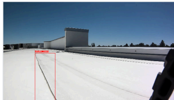
b Defective Seams (Medium)
