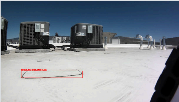
a Improper Equipment Supports (Medium)
